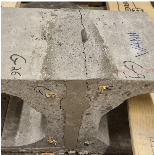
Figure 5.7: Crack has occurred
