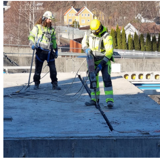
Figure 4.4: Open joint. Removal of residual joint with the use of a jackhammer
