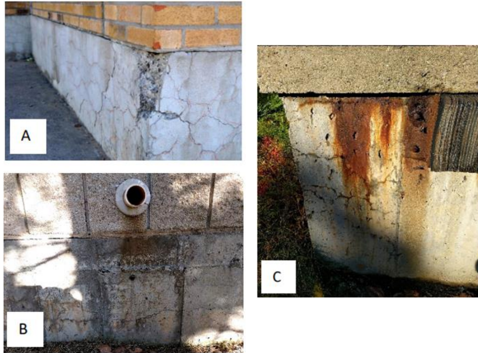
Figure 2.1: (A) and (B) examples of damage from the Trois-Rivières region. (C) damaged house foundation in Connecticut, USA. Figure taken from [12] and modified.
