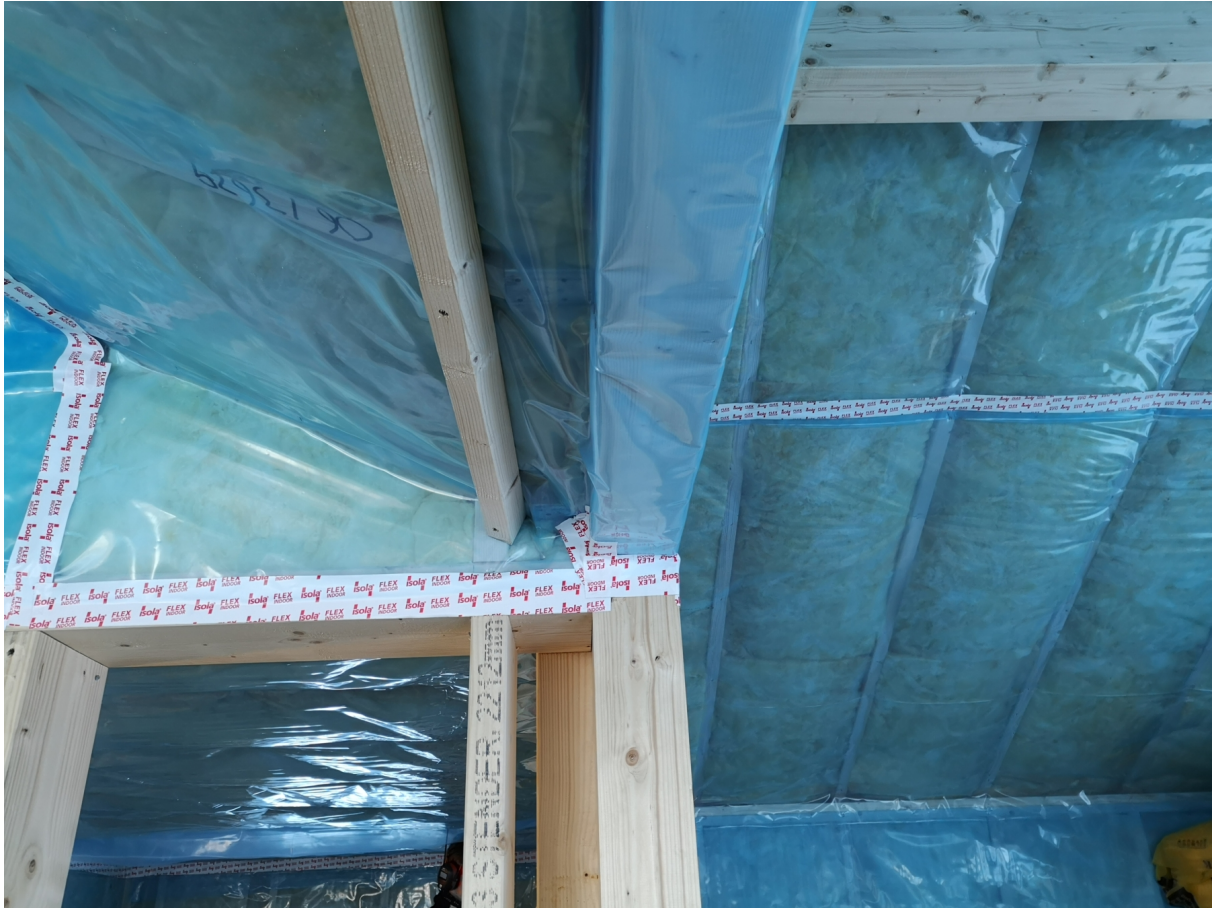
Figure 2.4: Adhesive tape used to join sheets of vapour barrier membrane, and to connect the membrane to the timber frame (Bygghjelp, 2019).
