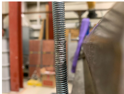
Figure 4.9.: Another damaged threaded rod
