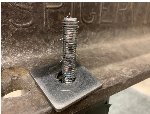
Figure 4.8.: One damaged threaded rod
