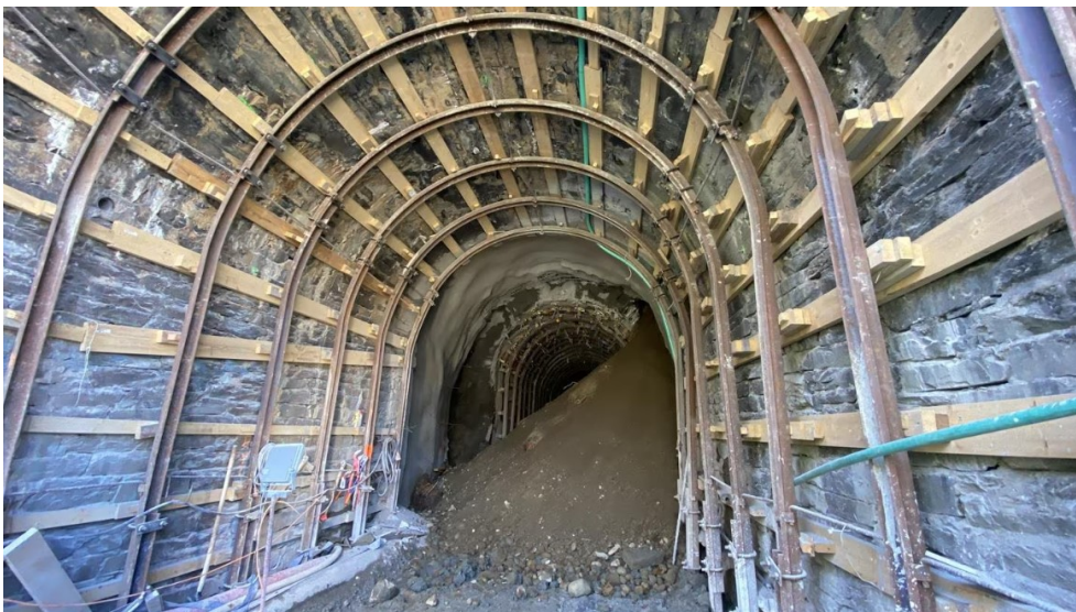
Figure 2.6: Picture of the avalanche in the Kronstad tunnel (Marita RamsvikKyrre Kjellevoid 2022).
