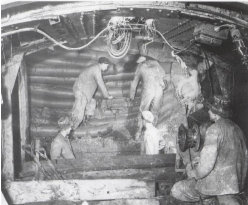
Figure 2.4: The picture was taken of workers digging out the clay at the face of the shield. The upper part of the shield can be seen in the upper part of the picture (Hansen 2016).
