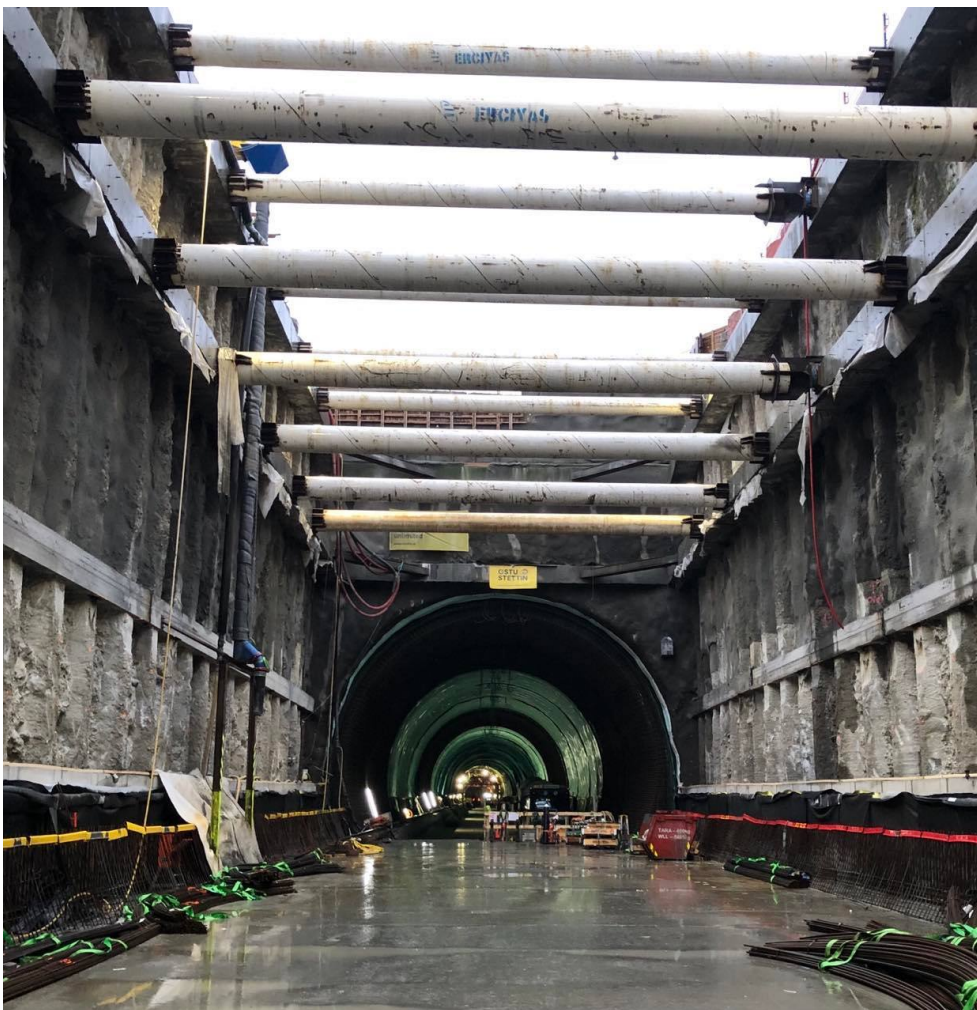
Figure 4.11: Picture of the entrance of the soft ground tunnel taken from inside the construction pit.
