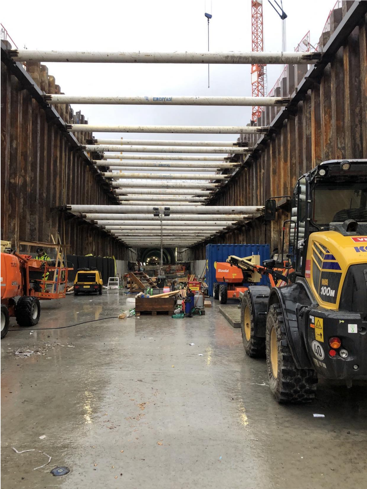
Figure D.1: Picture was taken from within the excavation pit at the site, 28.11.2022.
