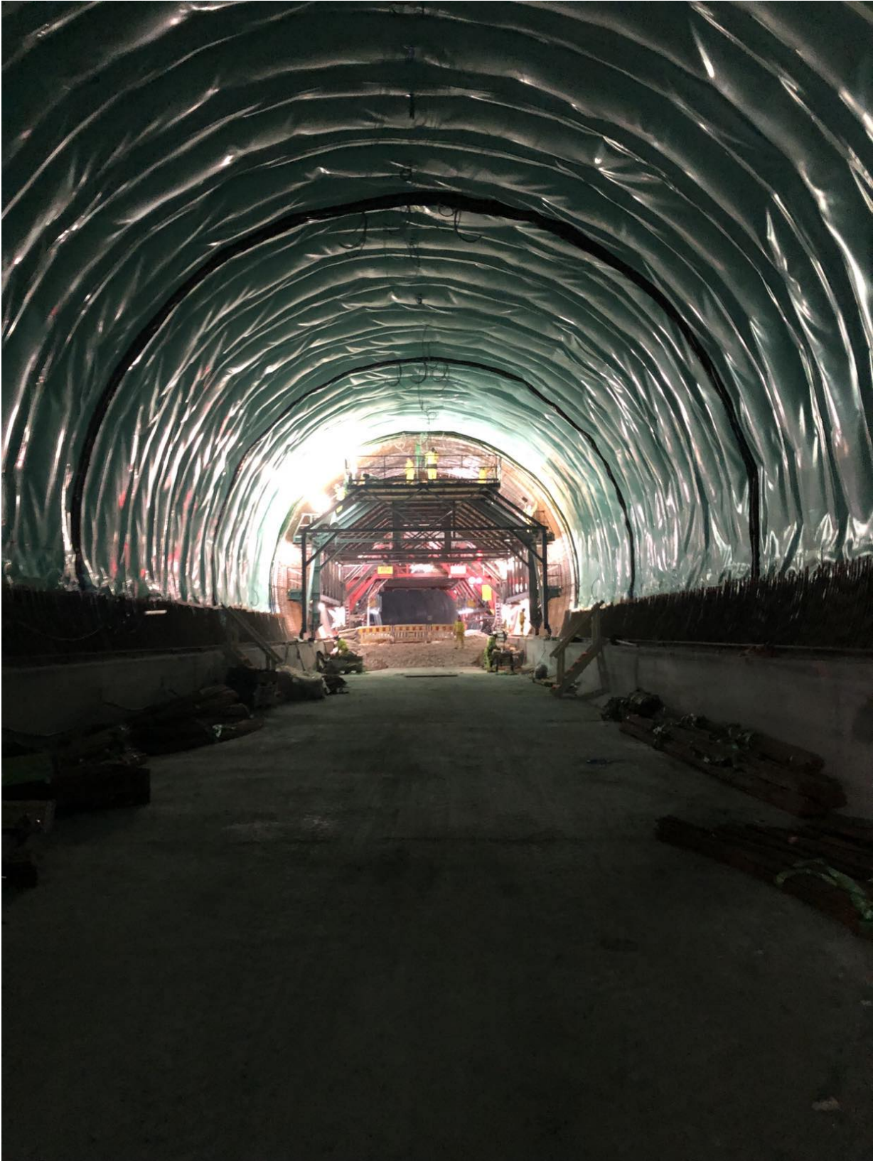
Figure D.3: Picture of the water sealing membrane, the permanent lining is being established in the distance, 28.11.2022.
