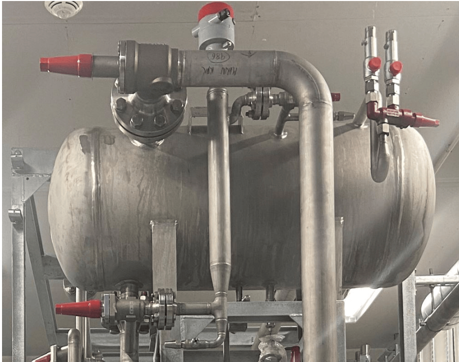
Figure 13: Liquid-vapor separator of the NTNU facility
