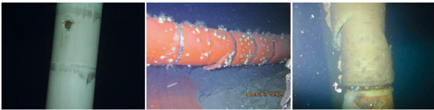
FIGURE 2.11. Example of external damage (ruptures) 25 © Anonymous Operator
