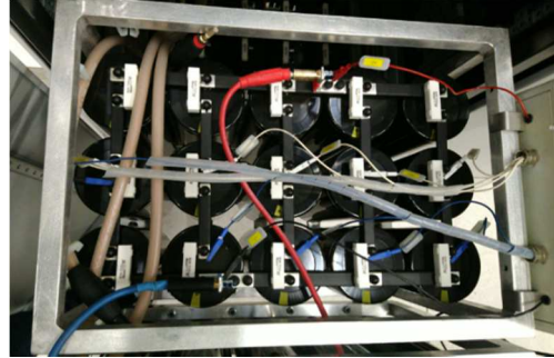
Capacitor Bank "B"
