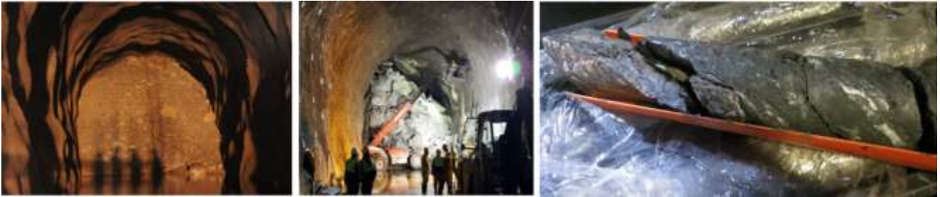
Figure 9. Collapsed tunnels passing through weak and weathered rocks of volcanic and sedimentary origin (left and center) and a cored highly weathered and weak flysch rock (right).
