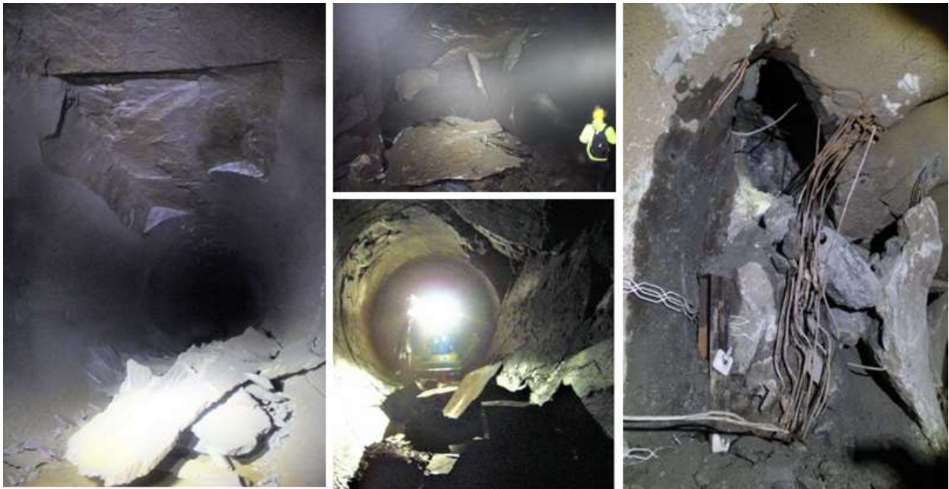
Figure 7. Examples of block falls and collapses witnessed in pressure tunnels and shafts of Norwegian HPP.
