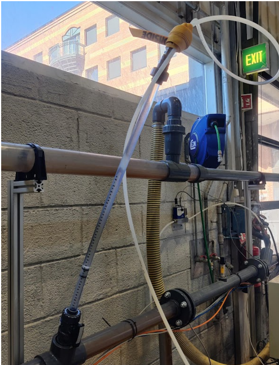
Figure 4.5: Sand injection system
