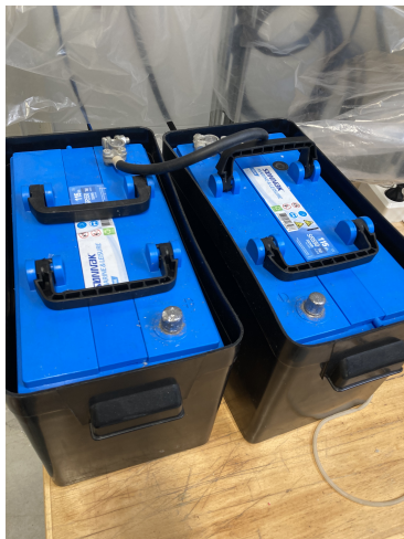
Figure 4.9: Original 12V batteries used for electrical storage in the system.
