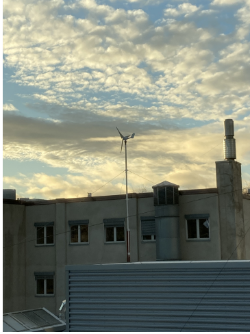
Figure 4.3: Original location of the wind turbine on the roof at NTNU.
