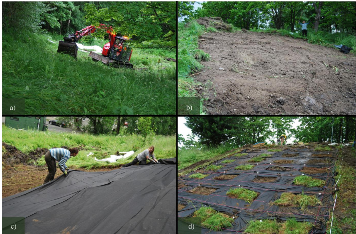
Figure A1: Stagewise procedure per grid: a) 8 park turf and 8 bulk were excavated. b) Remaining topsoil was stripped and excess soil from hole digging was placed alongside the grids, avoiding the control plot areas. c) Both grids were smoothed out with shovels, cleaned for rocks and remaining vegetation. The grid was covered with soil cloths four days later. d) Nine days in, all park and ex situ plots were inserted.
