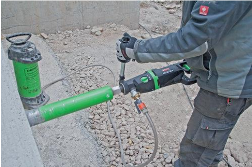
Figure 11: Core extraction of concrete (Eibenstock ETN 162/3 P, 3-Speed Wet/Dry Diamond Core Drill with Built-In Dust Extraction Port - Holes up to 8", no date).
