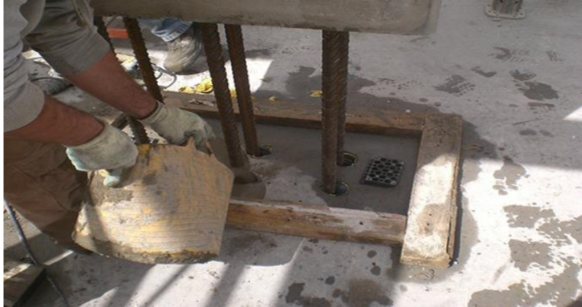
Figure 19: Installation of precast concrete column with coupling sleeves ('Reinforced Precast Concrete Columns', no date).
