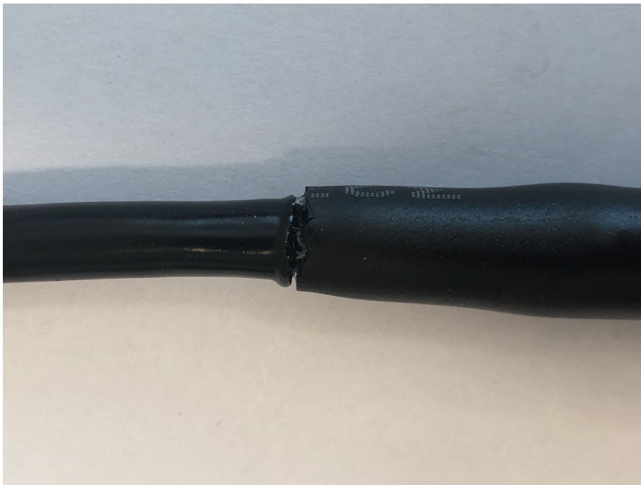
Figure 6.8: Deformation on cable after heat shrink.
