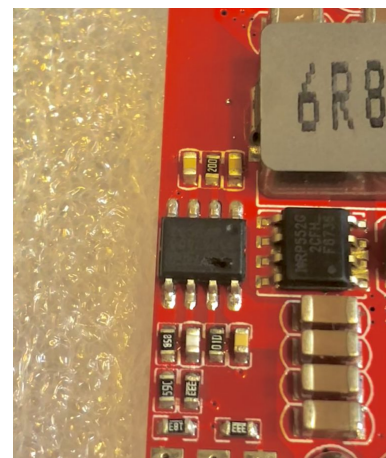
Figure 7.1: A hole in a component on the broken PSU.
