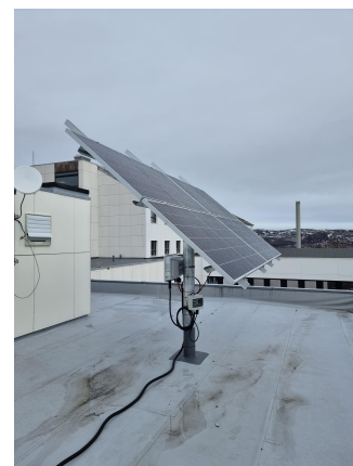
Figure 6.1: Test PV panels on the rooftop
