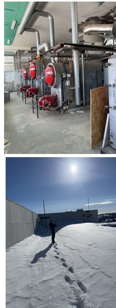
Figure 4.1: The visit to Kirkenes provided valuable insights, shown by the old oil boilers and the roof for the PV panels
