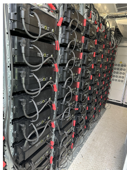
(a) Battery cells inside the container.
