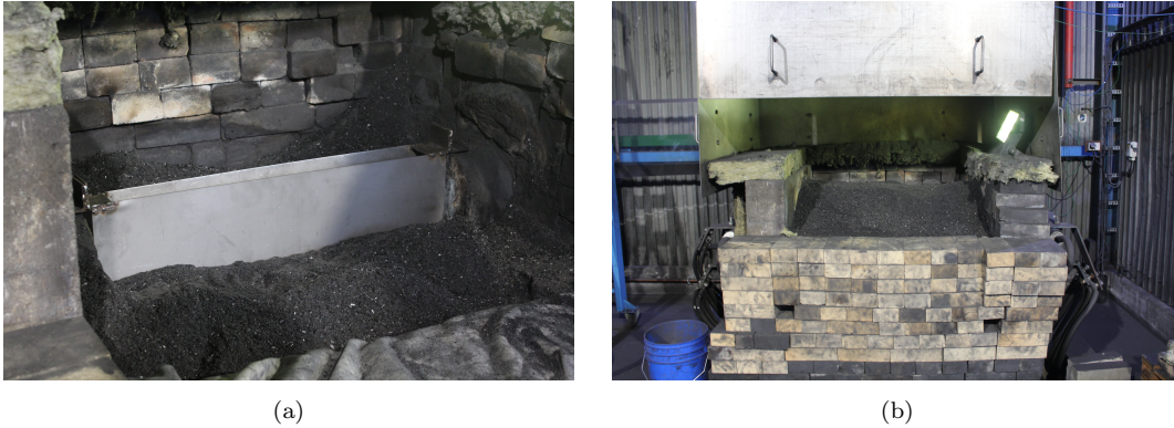
Figure 3.4: Building the pilot furnace. Steel insert for electrode (a), and finished furnace (b).
