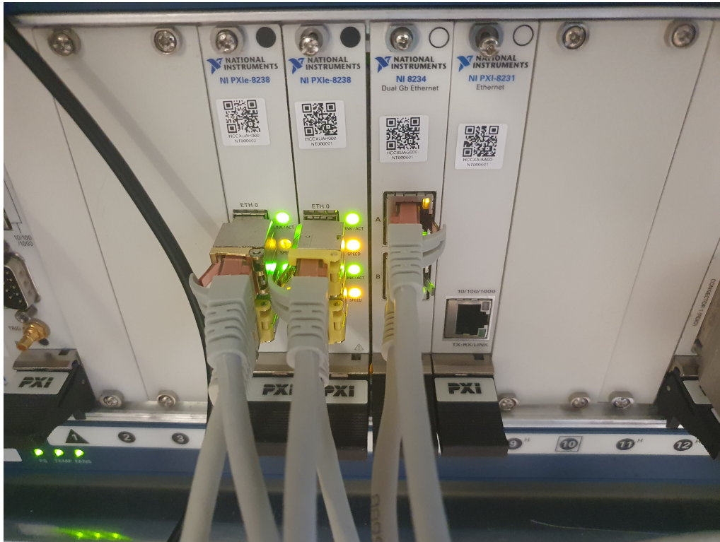
Figure 28: Photograph depicting the installed GbE expansion cards with 6 cameras connected via ethernet cables
