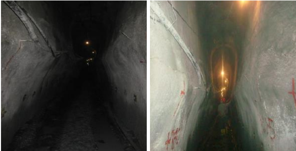
Figure 5-5: Squeezed tailrace tunnel section along chainage 390-410m dated 22 nd July 2013
