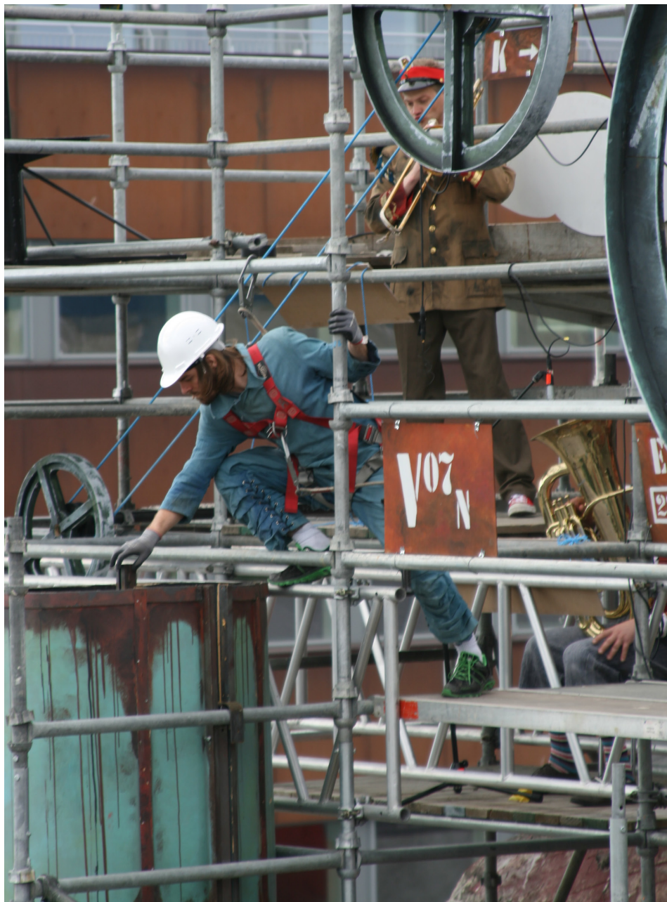
Figure 11: 'Harbour Happenings: The importance of being a stranger', 2016. Students work on the scaffolding construction as part of the staging of their projects, while musicians play in the background [Photograph: Johanna Gullberg. All rights reserved].
