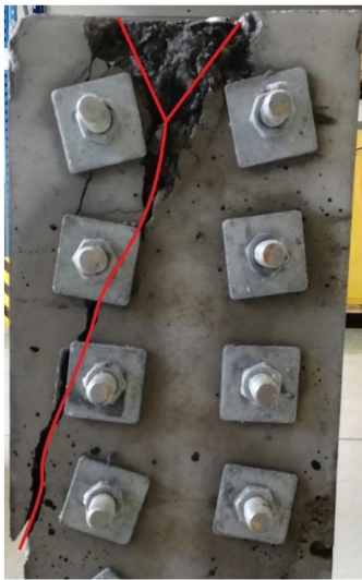
Figure 9. V-shape cracking pattern
