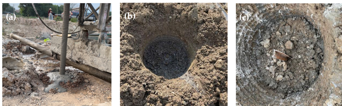
Figure 6. Influence of mixing times on oozing slurry of a mixing pile: (a) two, (b) four and (c) six.
