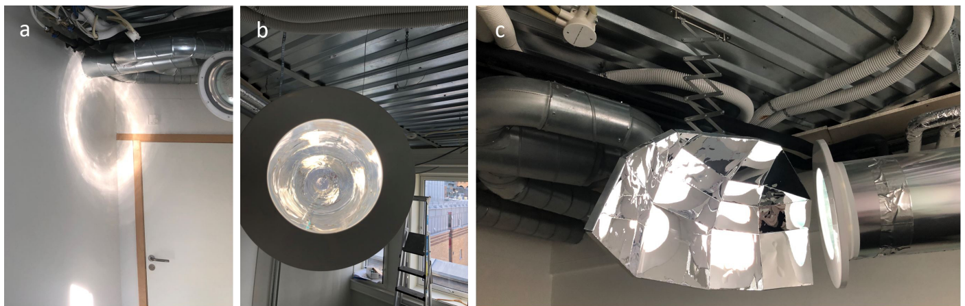
Fig. 4. Circular belt formed by light output from the HLP with clear transparent diffuser on the adjacent wall (2 m-distance) in January at noon (a); view of the light pipe opening, with mirror surface (b); custom-made reflector; the suspension is enabled by a scissor mechanism that allows for an easy adjustment in place (c).
