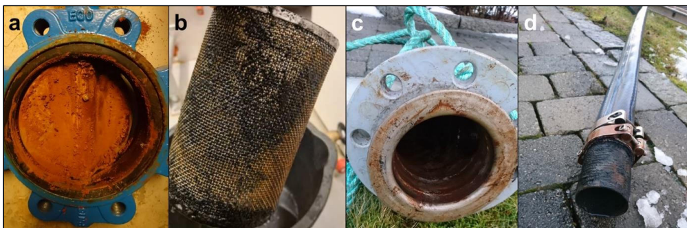
Figure 4.3 Incrustations sampled for a SEM analysis and b-d DNA sequencing. Samples from a replaced valve in groundwater pipe before heat exchanger at Lena terrasse, b groundwater pipe filter before heat exchanger at Buen, c top and d bottom of injection pipe (flexible hose) at Lena terrasse.
