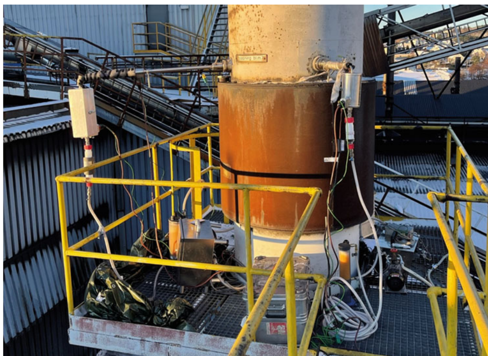
Fig. 2 Picture of the casting emission point with all equipment installed
