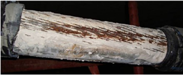
FIGURE 21 Example of whitish segregated grout embedding corroding strands in an Italian bridge 37
