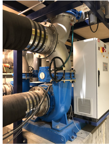
Figure 6.14: The valve that adjusts the inlet of the pump.
