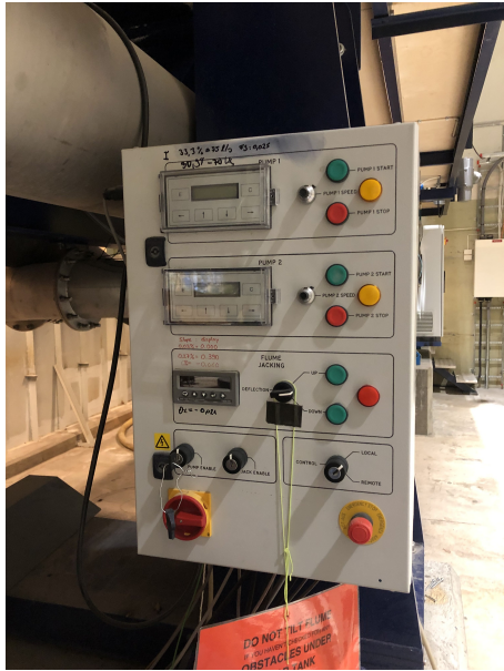
Figure 6.13: The panel where the pump is operated from.
