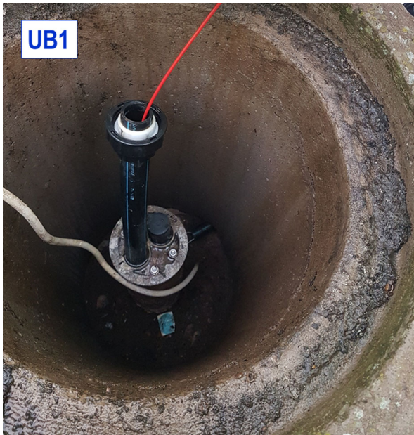
Fig. 4. Installation of optical fiber cable in the observation borehole UB1 outside the BTES.
