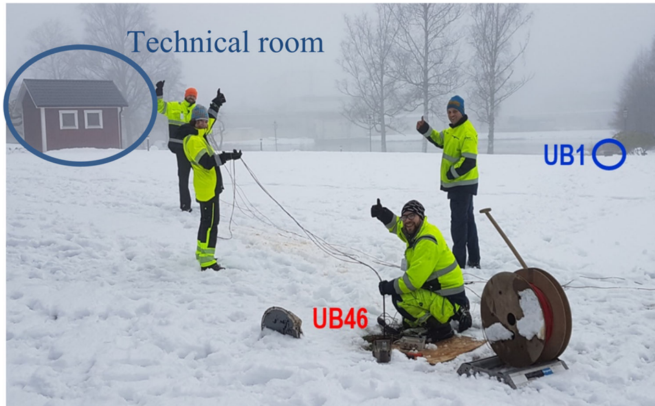
Fig. 6. Installation of fiber cable in observation borehole UB46 inside the BTES and location of UB1 outside the storage. Both fiber cables are lead through cable pipes and connected to the DTS system in the technical room.
