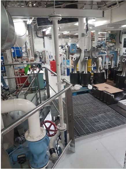
Figure 6. The engine room during an engine overhaul (Vessel 1).
