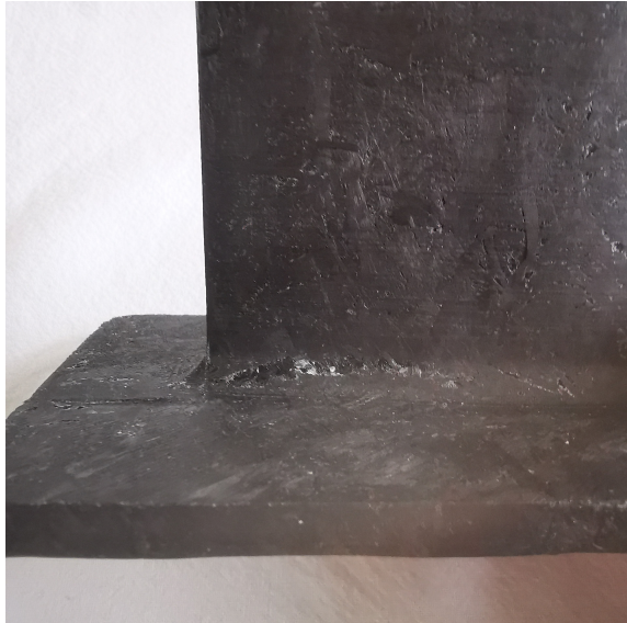
(b) A defect at the flange transition.
