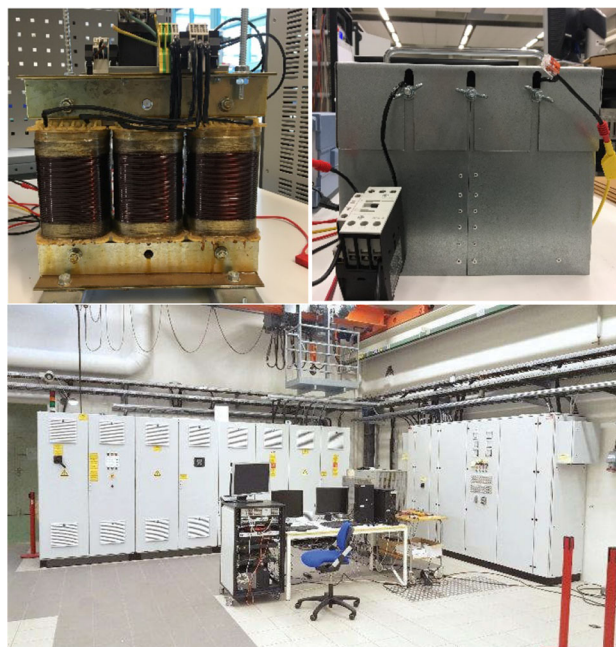
Fig. 5 Test setup. 2.5 kVA three-phase, three-limb transformer for dc-bias test with (upper right) and without (upper left) iron tank. The EGSTON grid emulator (in National Smart Grid Laboratory operated by Norwegian University of Science and Technology and SINTEF Energy) provides controllable voltage source (lower)
