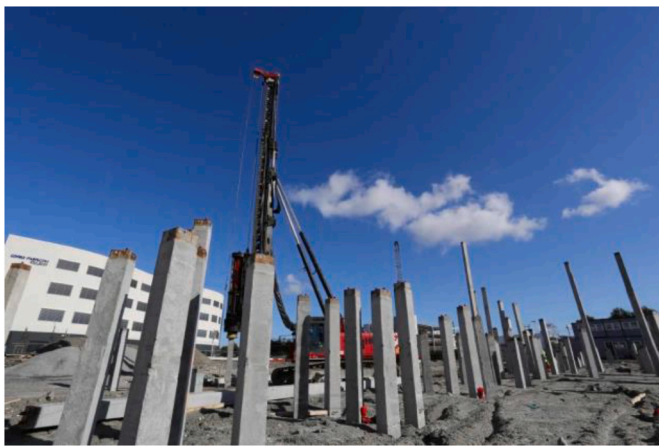
Fig. 23. A precast driven concrete pile project in Norway [Personal communication with Sandnes & Jærbetong company].
