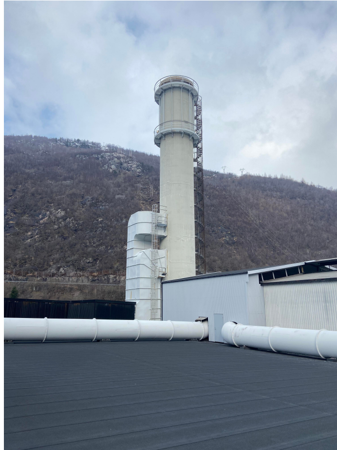
Figure 3.1.6: The wet scrubber of Hydro Aluminium Høyanger.
