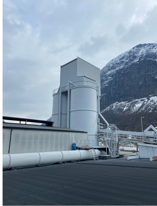
Figure 3.1.5: The dry scrubber of Hydro Aluminium Høyanger.
