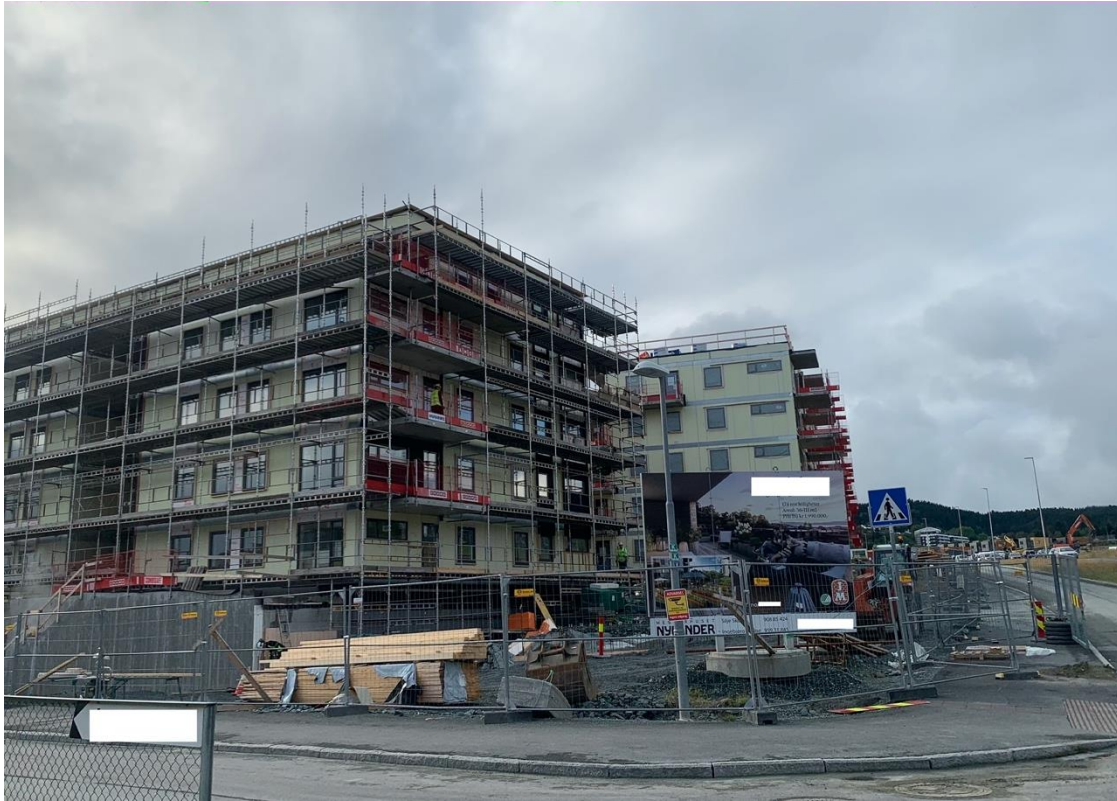
Figure 3.3 It was prohibited to enter the construction premise. View from across the street.
