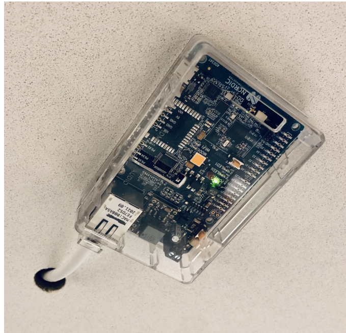
Figure 19: A PCA20036 kit mounted on a ceiling plate in the Trondheim office of Nordic Semiconductor. Each kit is enclosed in a Raspberry Pi casing for protection from dust.
