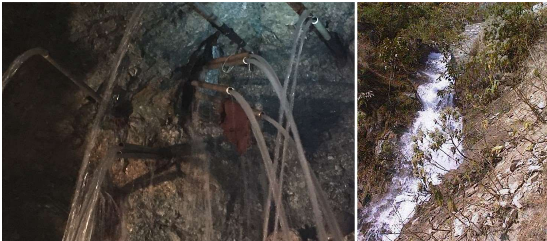
Figure 15. Water inflow in a headrace tunnel striking a weakness zone (left) and leaked water from a headrace tunnel during test water filling (right).
