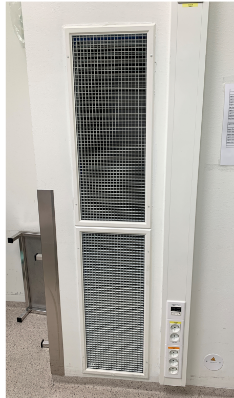
(b) Wall mounted exhaust vents
