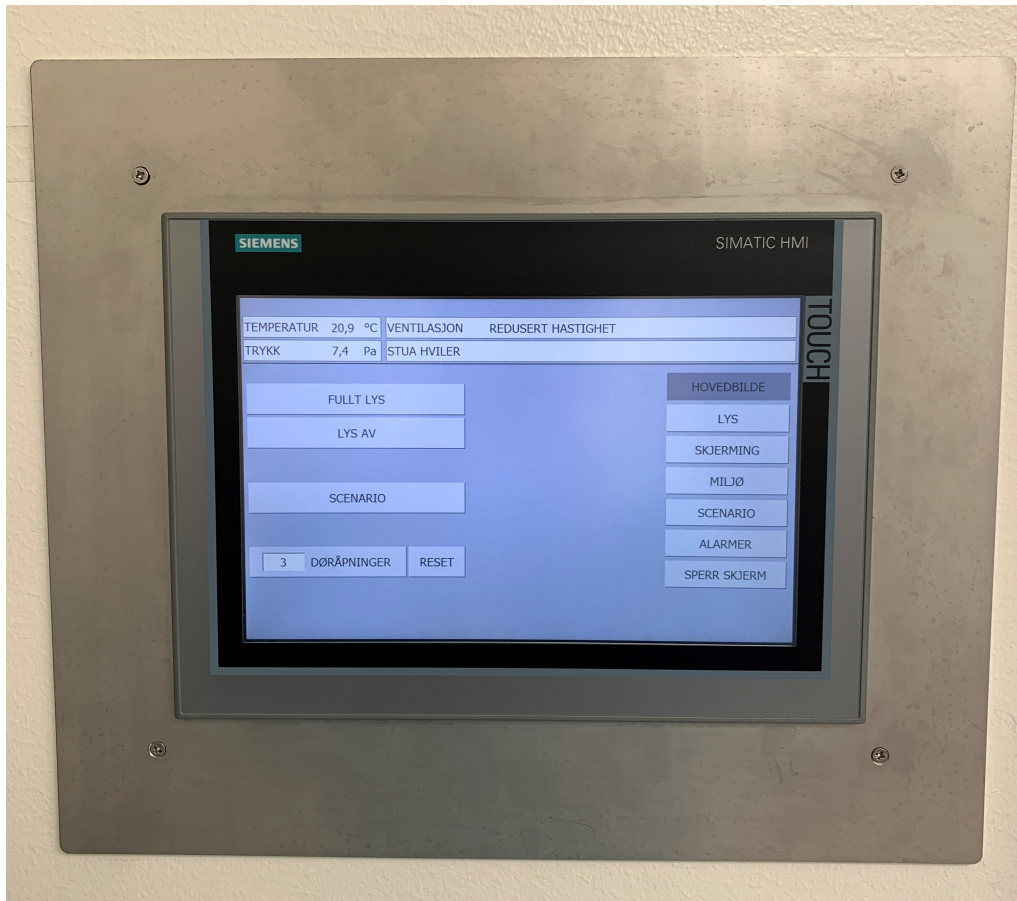
Figure 10: Indoor climate display in the operating room
