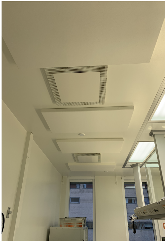
(a) Ceiling mounted exhaust vents
