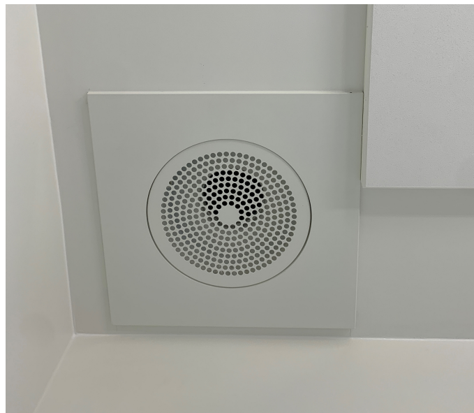
Figure 12: Ceiling mounted overflow exhaust vent placed in the north-east corner of the ceiling
