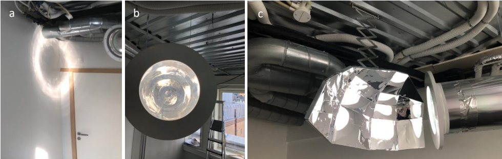
Fig. 4. Circular belt formed by light output from the HLP with clear transparent diffuser on the adjacent wall (2 m-distance) in January at noon (a); view of the light pipe opening, with mirror surface (b); custom-made reflector; the suspension is enabled by a scissor mechanism that allows for an easy adjustment in place (c)
