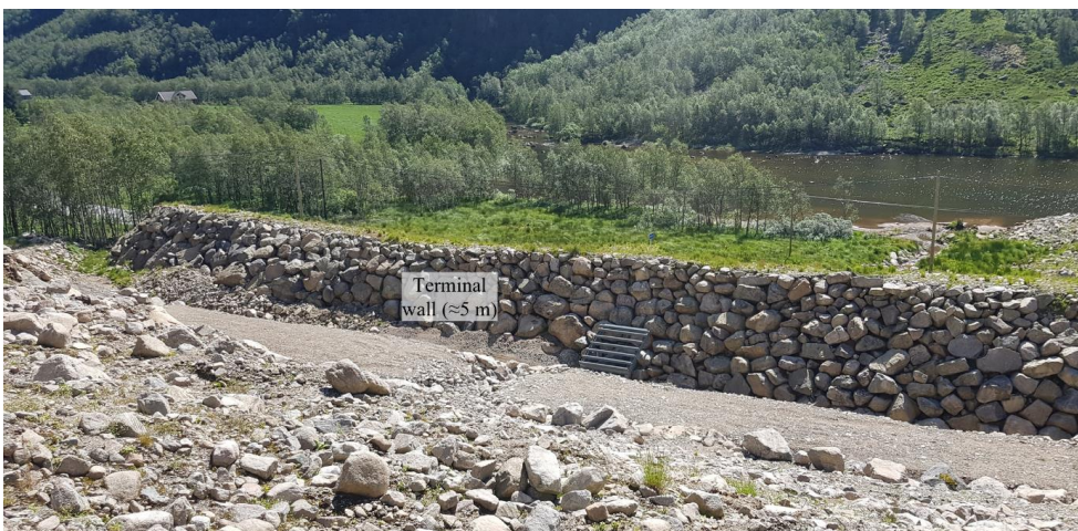
Figure 1.2 Terminal wall built in Hunnedalen after the debris flow event in June 2016 to protect the road against future debris flow events
