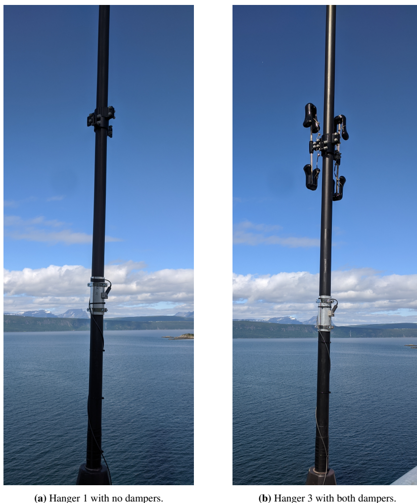
Figure 5.3: Damper and accelerometer installations on hanger 1 and 3 at the Hålogaland bridge.
