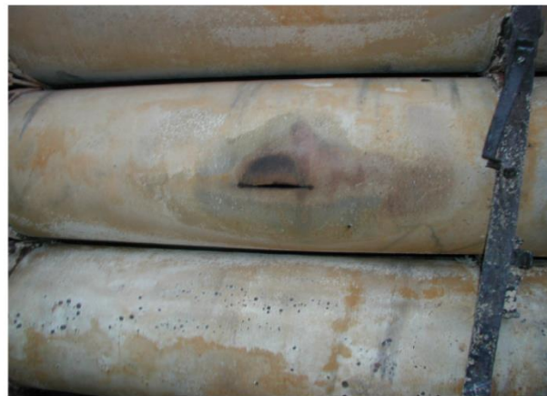
Figure 1.7: Longitudinal crack on one of the cylinders (Pilo et al., 2005)
