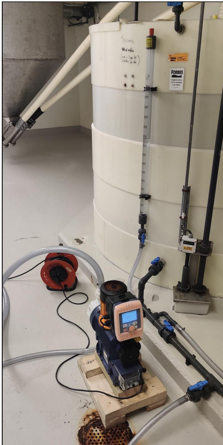
Figure 20. Membrane pump for pumping salt brine from the brine tank to mainline at VIVA
