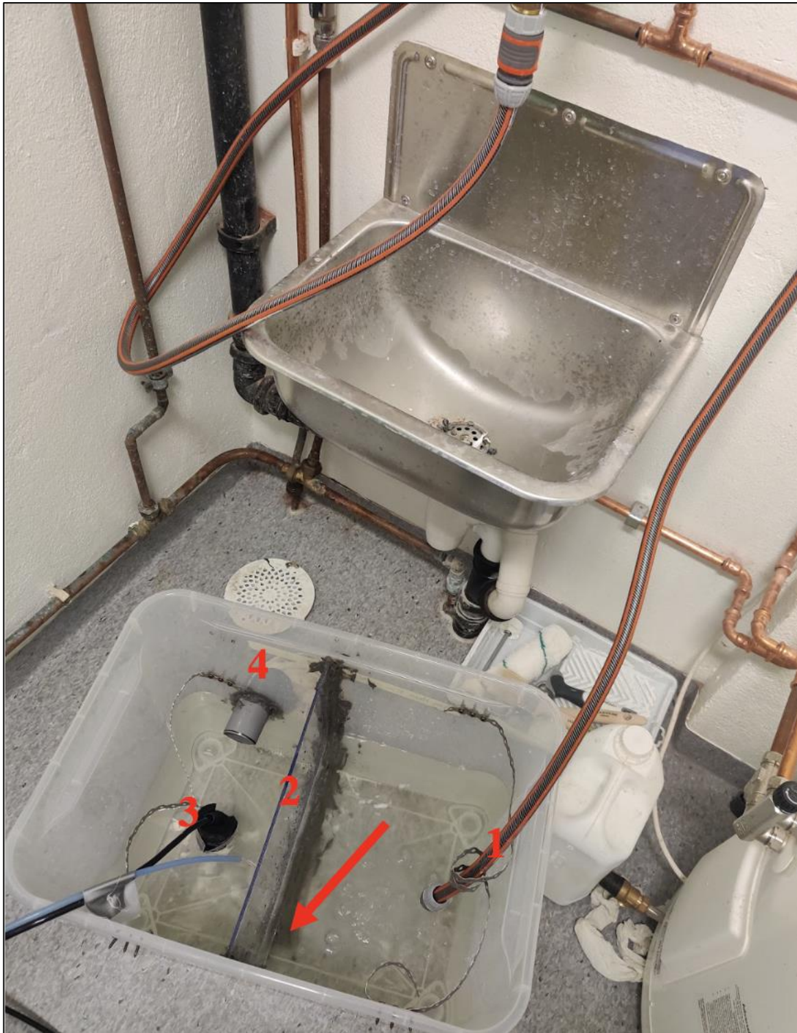
Figure 19. 70L plastic box at Jakobsli pumping station. 1. Inflow from faucet connected to a hose. 2. Separation wall. 3. Conductivity probe. 4. Plastic outlet pipe. Red arrow points to the opening in the bottom of the box that connects the inflow chamber to the measuring chamber.
