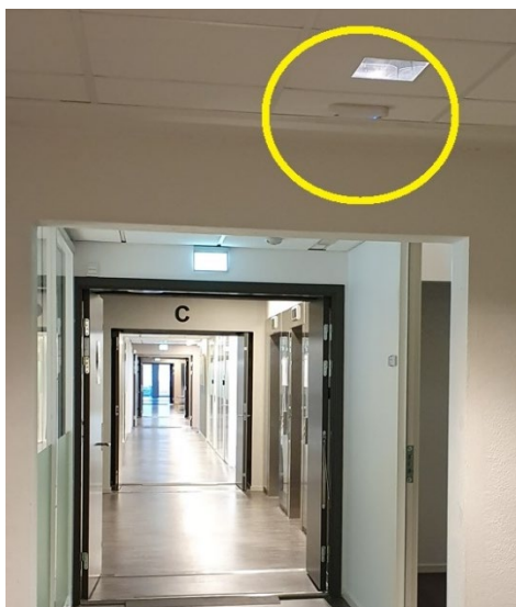
Figur 4.1: "Footfall" sensor montert i tak
