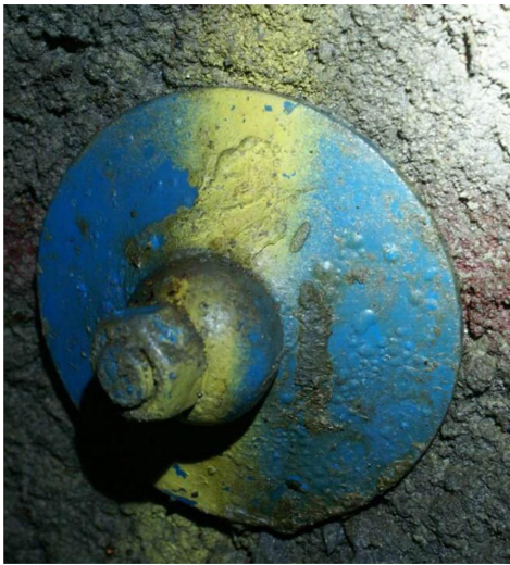
Fig. 12 Blisters observed in the rock bolt plate in the Oslofjord sub-sea road tunnel after 10 years of exposure (Ongstad 2012)
