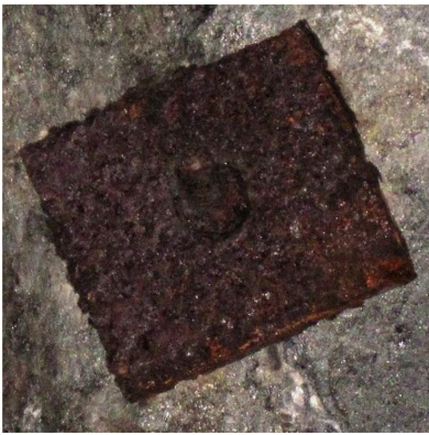
Fig. 4 Fully grouted uncoated rebar with unprotected steel accessories in the Hamregjøel tunnel after 47 years in service (Ongstad 2012)
