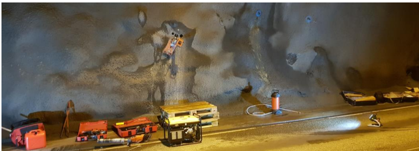
Fig. 4: Three shotcrete cores already extracted in the Frøya tunnel at chainage 8+070 near the north portal. The corresponding extracted cores are shown in paper 3, Fig. 5.
