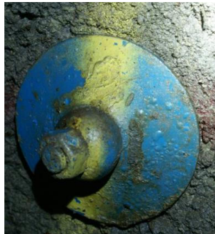
Fig. 18: Blisters observed in a rock bolt plate in the Oslofjord subsea road tunnel after 10 years of exposure [61].
