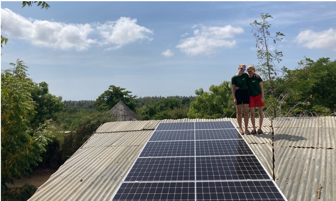
Figure 18: PV panels of the new PV system installed on the roof of Class 5.
