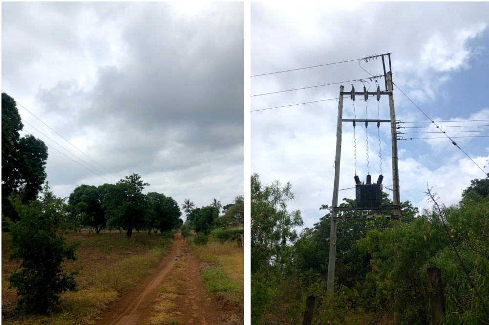
Figure 17: The transformer closest to Eco Moyo and the local grid with three phase wires.
