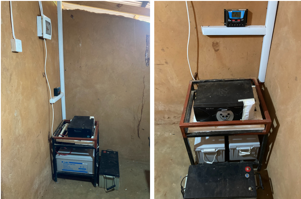
Figure 19: System at kitchen.
