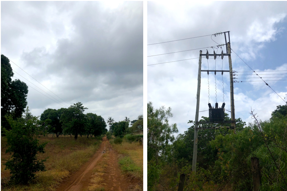
Figure 17: The transformer closest to Eco Moyo and the local grid with three phase wires.
