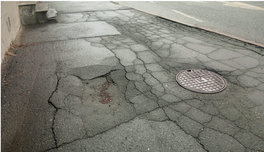
Figure 13: Damaged pedestrian pavement [Photo: by author]
