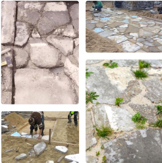
Figure 22 Irregular shaped fragments of demolished concrete from a residential building built in 1959, being reused on site to cover the ground of the outdoor spaces. Clos Saint Lazare in Stains, France, 2017. 56
