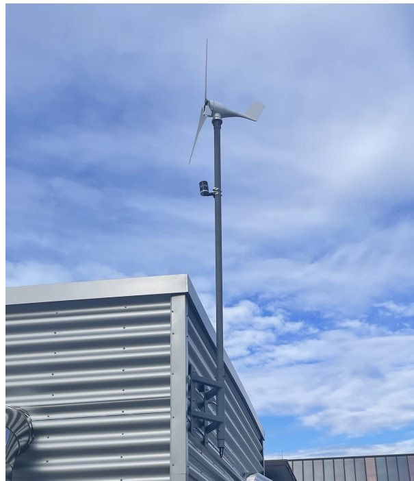
Figure 4.26: Location and mounting of the wind turbine on top of the technical building on the roof of the Thermal Laboratory.
