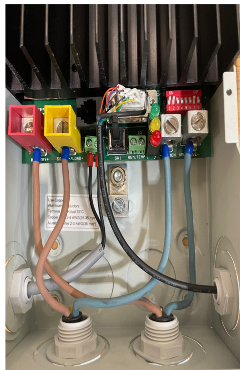
(b) Wiring of the controller, the DIP switches can be seen in the upper right corner.
