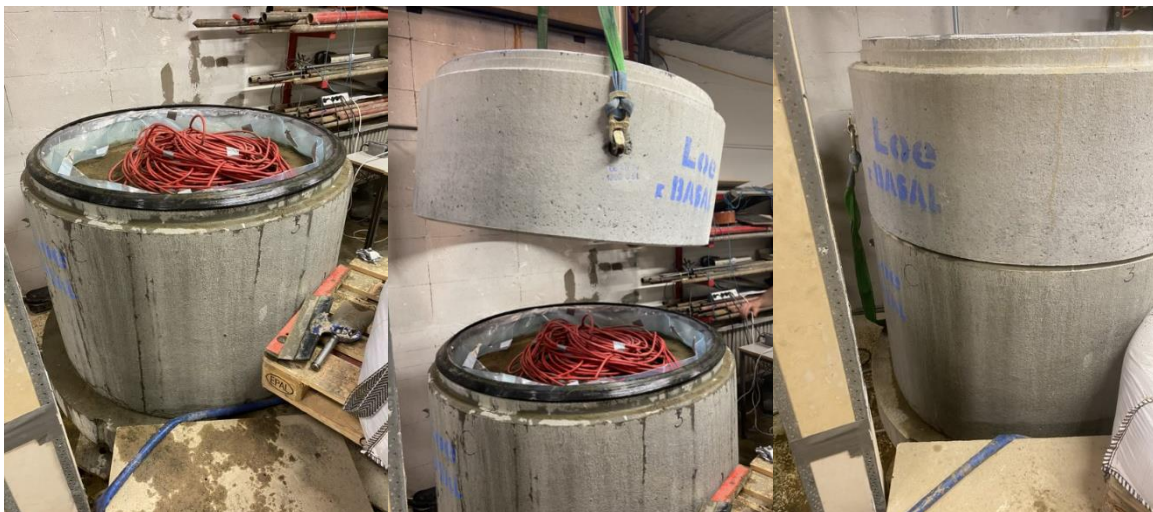
Figure 6: The extension chamber element is hoisted down and placed on the cottom chamber.
